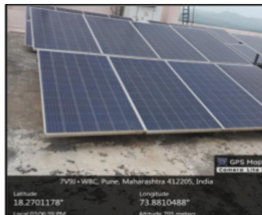
Photograph of Roof Top Solar PV Plant:
